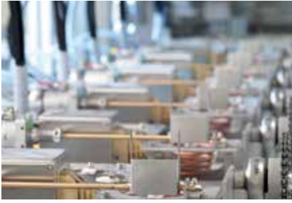
Row of fusion units ready for operation.
